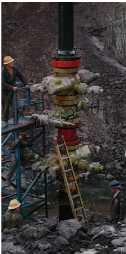
After the well is capped, workers nipple up the BOP stack and diverter lines. Photographs courtesy of ALERT Disaster Control.
