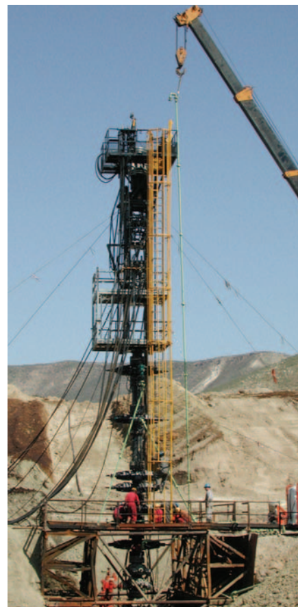
Here the snubbing unit is rigged up following complete recovery operations. Photograph supplied courtesy of ALERT Disaster Control.
