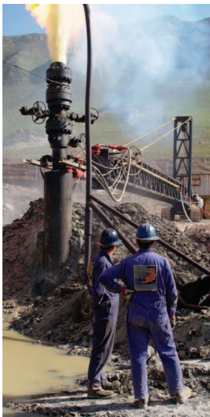
Preparing for abrasive jet cutting operations with the ALERT Hellcat/Athey wagon. Photograph courtesy of ALERT Disaster Control.
