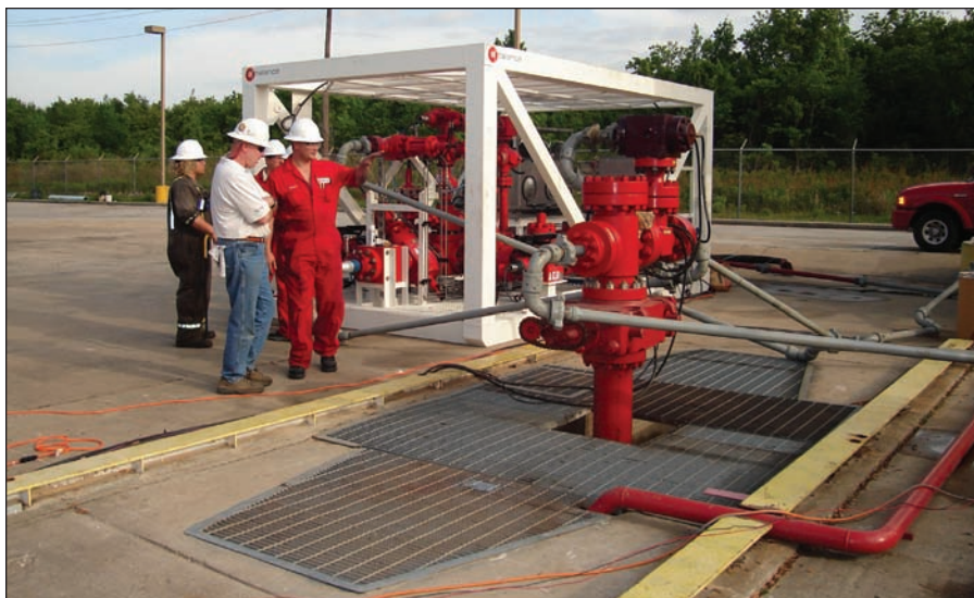
IADC/SPE 112662: Shell E&P continues to successfully execute redevelopment slimhole sidetracks using MPD on the Auger TLP in deepwater Gulf of Mexico. Above, MPD equipment is tested for offshore use.
