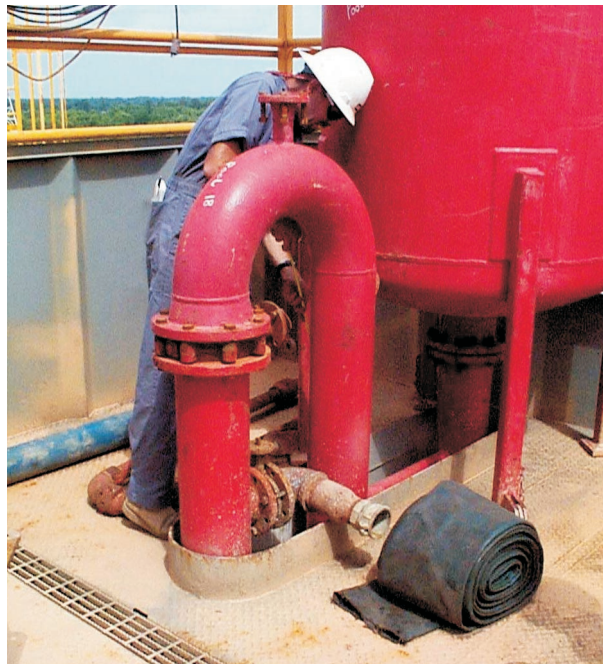
A technician checks out the length of the U-tube on a mud/gas separator to determine if it will be able to handle the required flow.
