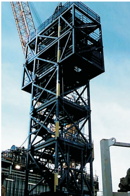
Coiled tubing drilling tower, shown installed on platform, is designed for safety and flexibility.
