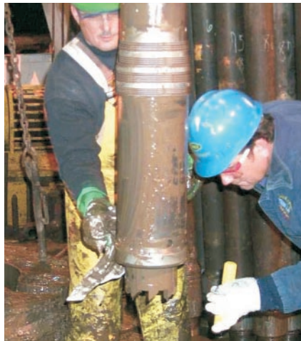
Expansion cone (mandrel) is coming out of the hole on the first offshore SET installation.
